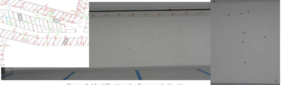
Figure 4: Identification des fissures et situation
